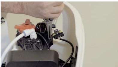
Water inlet filter replacement
